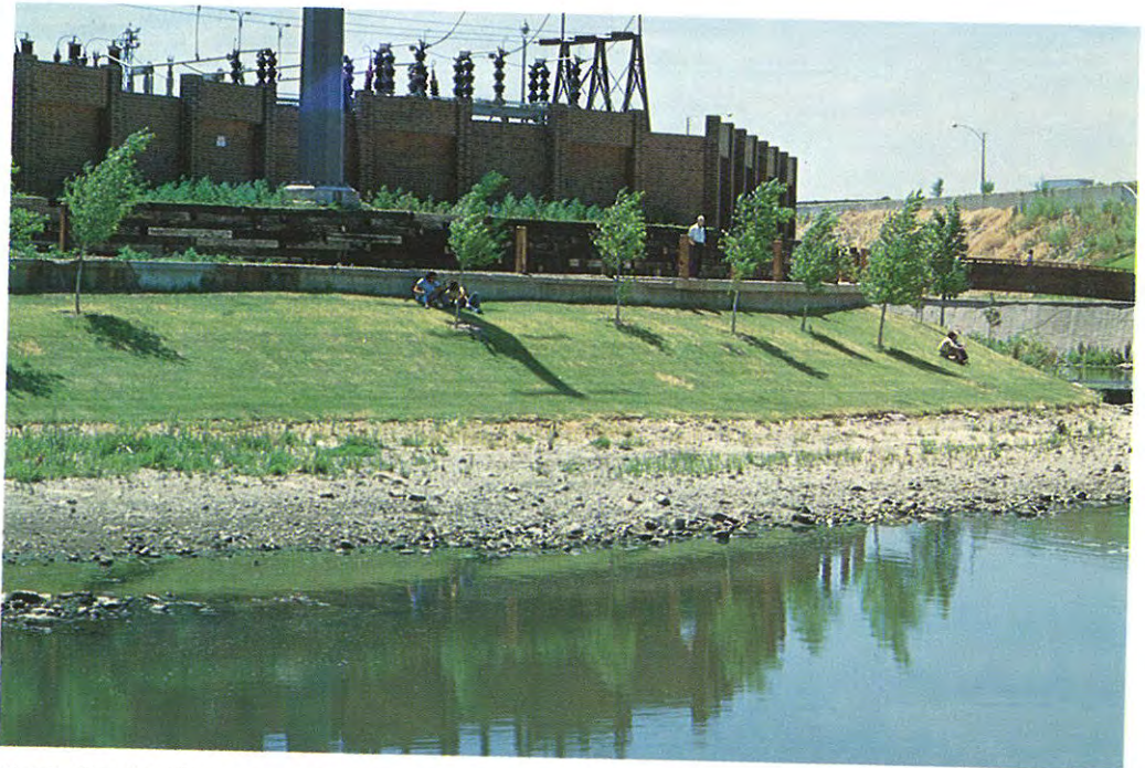
Public Service Company substation after improvements by Company and by Committee (restoring riverwall, trees and grass).
