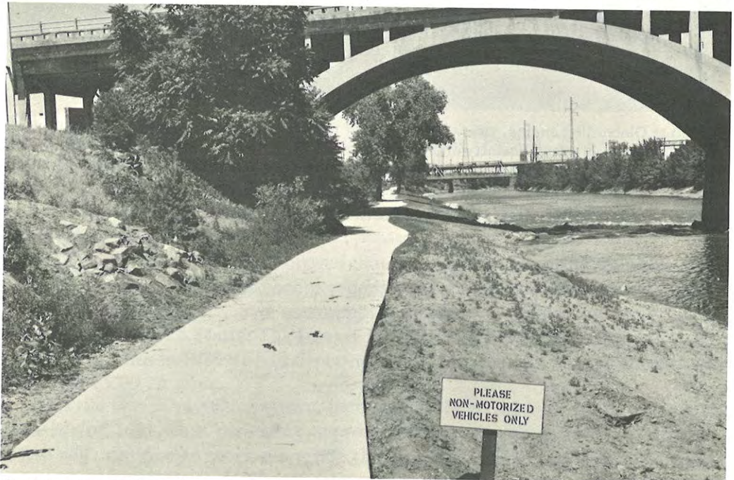
Section of concrete trail, ready for sweeping, looking downstream (north) through 16th Street Viaduct toward 19th Street Bridge and 20th Street Viaduct.
