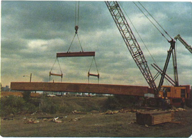
One half of wooden bridge located north of Florida Avenue being lifted into place.
